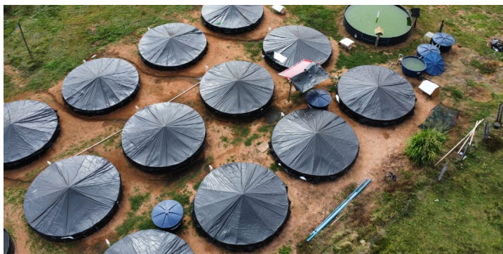
Tanks installed in a rural settlement
